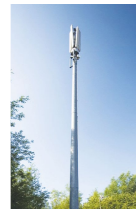
Antenna & StreetPole Masts
